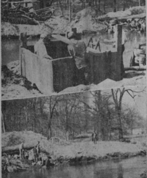
Markings on the top photo are showing a contractor for the first pier of the new toll bridge... Fleetwood toll span... Construction work...
