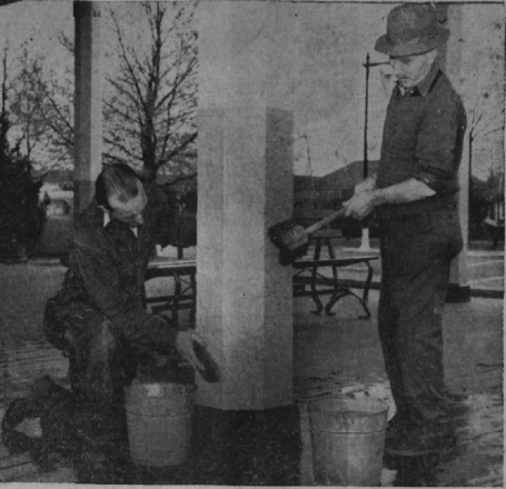
Workers are shown yesterday as they helped fix Playland, Westchester's amusement center at Rye, for its "Grand Opening" tomorrow. Incidentally they're saving taxpayers quite a few dollars by substituting elbow grease, soap and water for paint in making the park shine like new.
