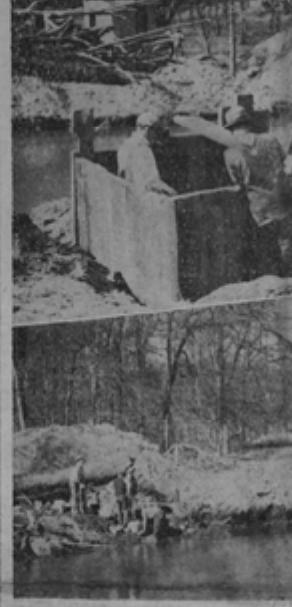
Workers on the top trestle are sinking a railroad for the first pier of the new toll bridge to parallel the present Veterans span which makes a bottleneck in the heavily traveled New York Parkway. Plans are being made in the meantime to decide what type of foundation must be used. Before the contract is let, the bridge has been changed to facilitate work on the pier.
