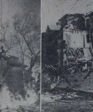
Debris is shown burning in left photo while a closeup of the partially demolished house is shown at right. A two-story frame cottage at rear, formerly owned by the Parks estate, was burned yesterday when workmen didn't even bother to demolish it.—Staff Photos by Danie Raffail.
