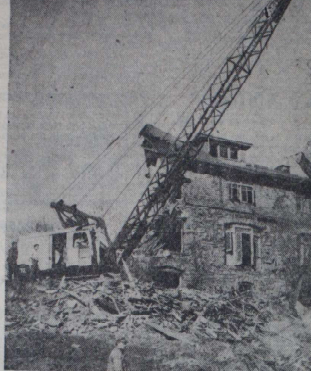
DEMOLITION of 145 Haven Convent Home by a large crane to make way for the Thruway construction along the Bronx Post Road.
