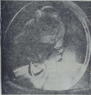
"DOUBLE RING" CEREMONY —It's a case of "to have and to hold" in this "double ring" ceremony at the East Pittsburgh works of the Westinghouse Electric and Manufacturing company. The upright ring is having an arc welding treatment to join its ends in a perfect circle, while a similar ring, atop still other rings, serves as a means of holding the welded object in proper position for the welder. The rings are rims for war-vital 500-horsepower motors.
