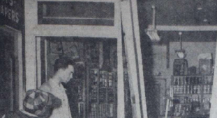
The wrecked shop window of a paint and wallpaper store at 436 Mamaroneck Avenue.
