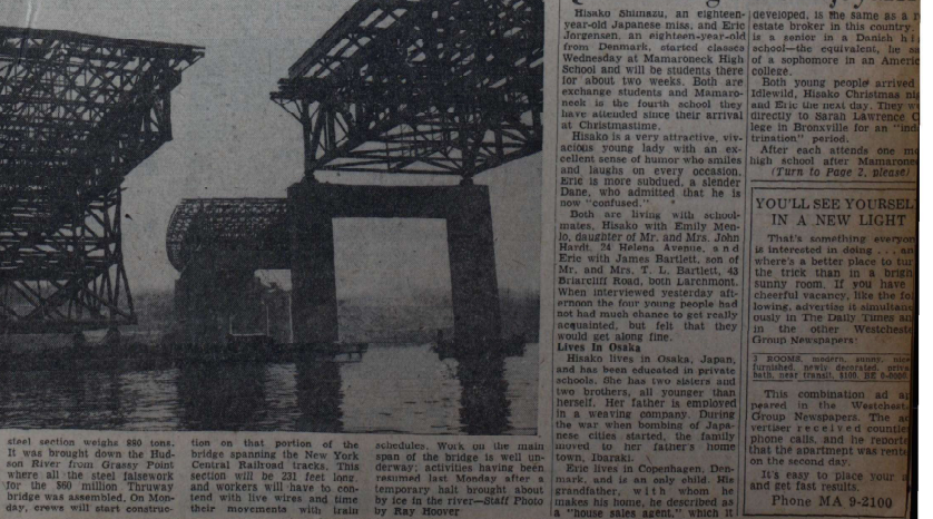
Steel section weighs 880 tons. Work on the main span of the bridge spanning the New York Central Railroad tracks. This section will be 211 feet long and workers will have to contend with live wires and time their movements with train schedules. Work on the main span of the bridge is well under way; activities having been resumed at Mamaroneck after a temporary halt brought about by ice in the river. Staff Photo by Ray Hoover.
