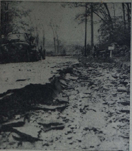
FLOOD DAMAGE to roads and bridges estimated in excess of $300,000 northern Westchester towns have launched a cleanup and repair job. Typical of the trail of destruction spreading from Cortlandt to North Salem is this scene on Trinity Pass Road in Round Ridge where Highway Department crews are filling in a major washout — Staff Photo by Warren Ingless
