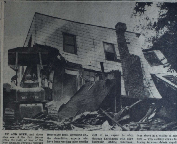
UP AND OVER, and down goes one of the first houses along the right way of the New England Thruway through Larchmont on Byron Place, Benvenuto Bros. Wrecking Co. demolition experts who have been working nine months on the job.
