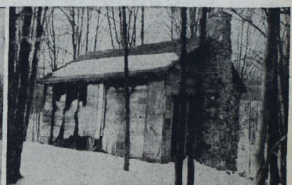
CAMP COOK'S QUARTERS —This building is nearly in the same condition as the camp director's cabin. Door, windows and flooring will have to be renewed, and other minor repairs made to render the place livable. It was built by Troop 21 of Oastling.
