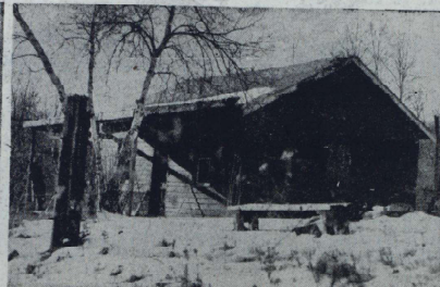
NATURE LODGE —Troop 21 of the Hastings-on-Hudson Boy Scout Organization originally built this shelter. It will need extensive repair. Set apart for nature study by Scouts, it will contain the nature-library and collections of mounted insects and stuffed birds and animals.
